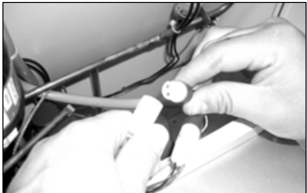
Fig. 72: Disconnect the fan connectors (3)
